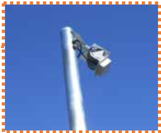
Antenna section of the units
