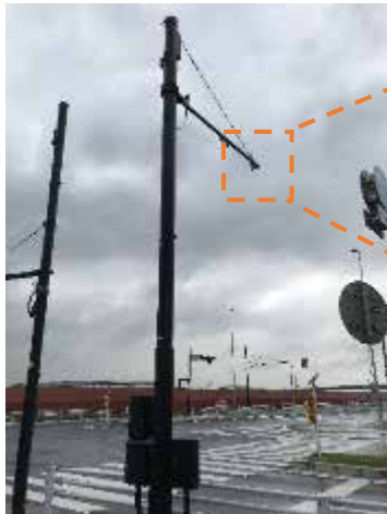
ITS wireless roadside units
