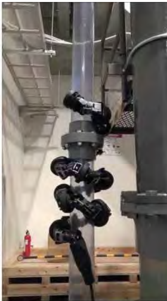
Outside of Pipe
