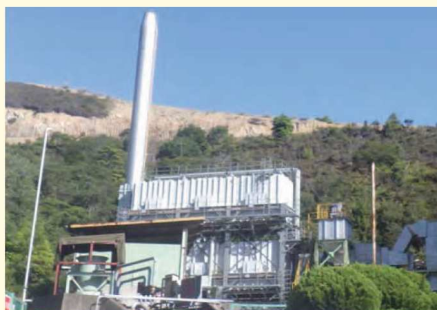
• Large-scale combustion test plant
