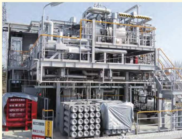
• Appearance of the pilot plant for ammonia production
