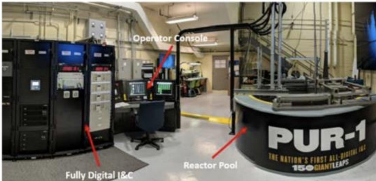
Figure 4: PUR-1 reactor room.
