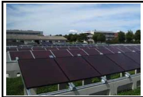
Photovoltaic Power Generation
