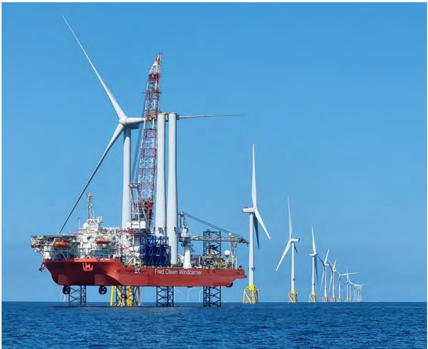
Moray East Offshore Wind Power Generation Project (UK)
